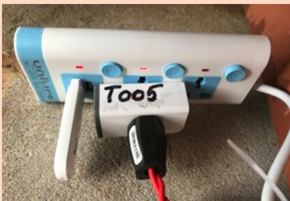
Power meter system
